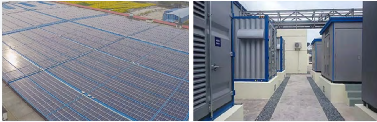
IKEA's first distributed PV project in China
