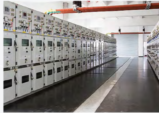
Power Distribution Project
